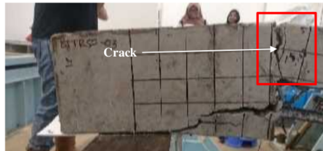
Figure 1. Cracks in the support zone.
